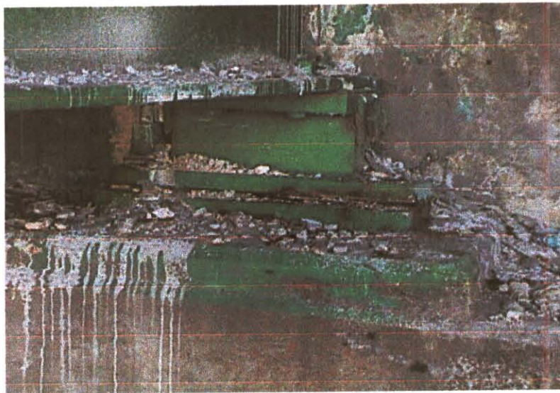
MISSING ANCHOR BOLT AT BEARING "A" ABUTMENT #1
