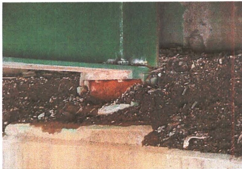
DEBRIS ON CAP COVERING BEARINGS ABUTMENT #1
