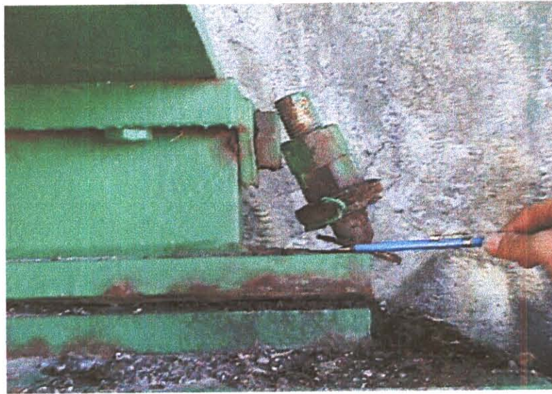
BROKEN BEARING BOLT BEAM "A" ABUTMENT #1
