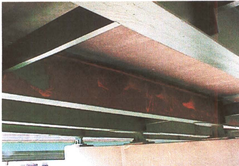
RUST BEAM "C" SPAN #3-TYPICAL
