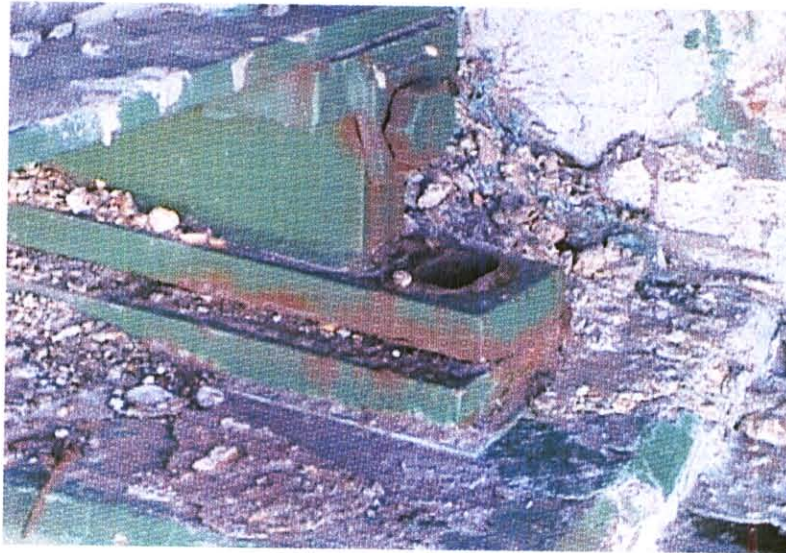
BOLT MISSING FROM BEARING "A" SPAN #1
