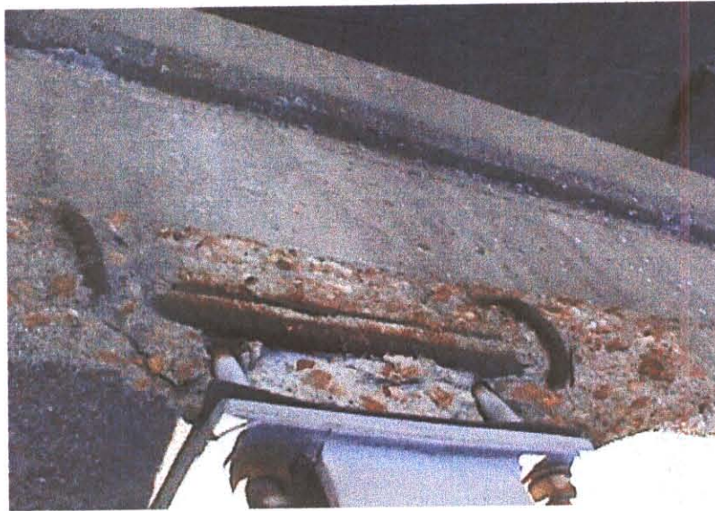
BREAKOUT WITH EXPOSED REBAR AT GUARDRAIL POST LEFT SIDE SPAN #
